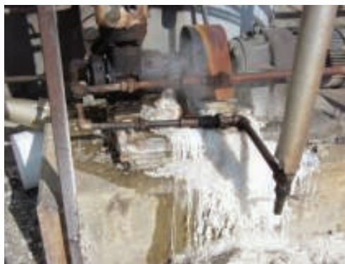
FIGURE 3. When leaks occur, valuable raw materials and end products are irretrievably lost, while the safety of plant personnel and the environment is put at risk. Damage is also done to the operation in the form of expensive costs for cleanup, downtime, parts replacement or the purchase of a brand-new pump
