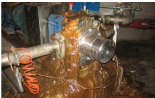
FIGURE 2. A shortcoming of mechanically sealed pumps in the CPI are the catastrophic failures that can occur when the seals fail, potentially causing dangerous leaks
