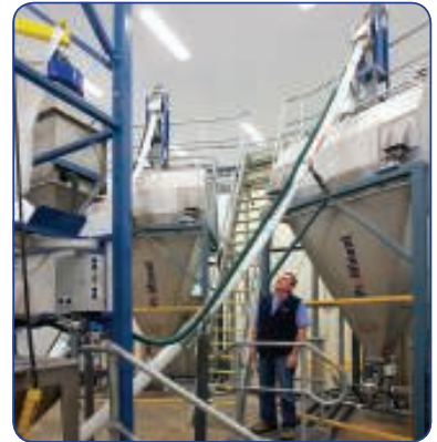
Two flexible screw conveyors feed fluoride powder from a bulk bag discharger into two seven-day storage hoppers
